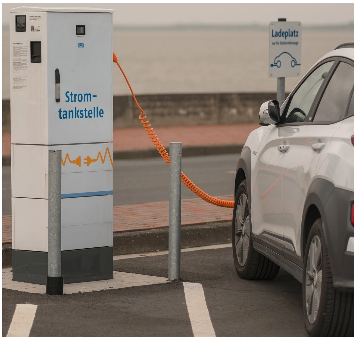
Car Charging Station
