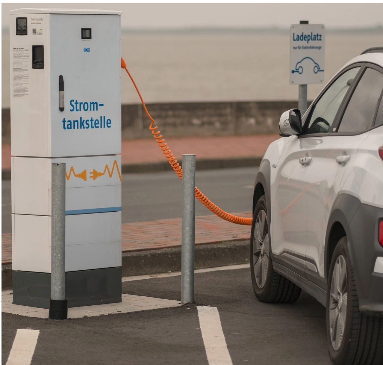
Car Charging Station
